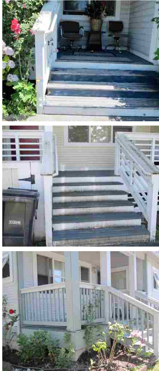
Image 22: First Two SHA-Rental Units' Porch and Stair Material Wearing and Deteriorating Compared to a Market-Rate Unit's Porch and Stair Materials with Better Quality (Third Photograph)
